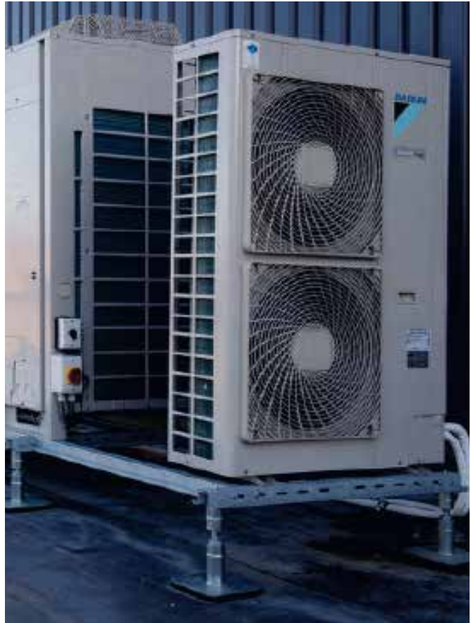
Air source heat pumps can be located on the topmost rooftops.
